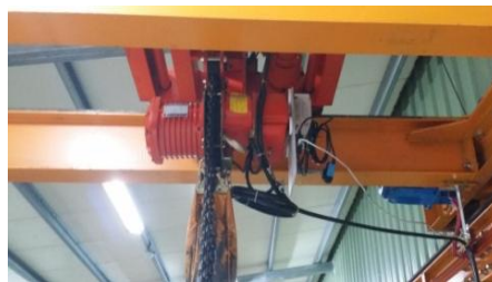
Figure 1: Side view of installation location of video monitoring module.
